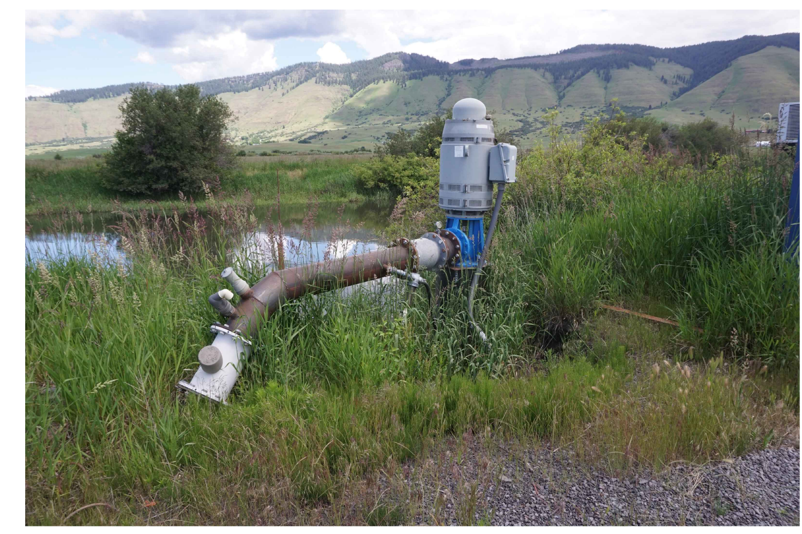
EXISTING VERTICAL TURBINE PUMP
